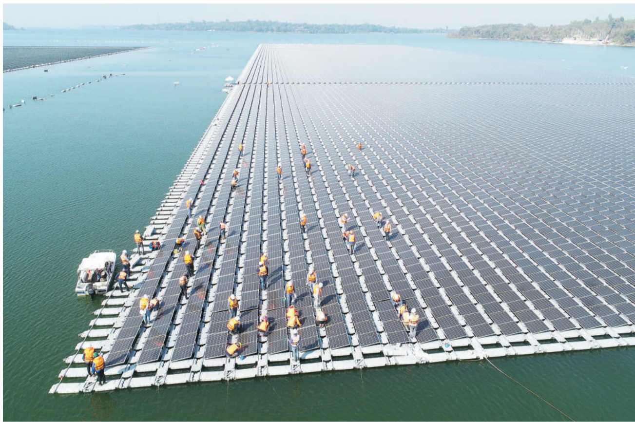
Construction workers checking the installation of floating solar panels at Sirindhorn Dam in Thailand's northeastern province of Ubon Ratchathani. The project is jointly constructed by China and Thailand. (PHOTO: XINHUA)
